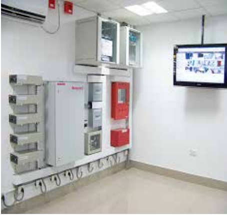
Server Farm Area of West Bengal State Data Centre
