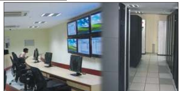
Inner View of Data Centre and Rack Area
