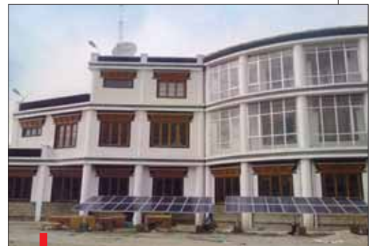
10Kwp Solar Power Plant installed at NIC Leh (IT Enclave)
