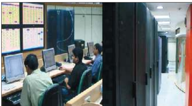
Inside view of Internet Data Centre and Communication Racks & SAN Storage at NIC (HQ)
