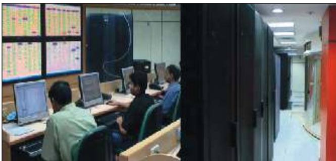
Inside view of Internet Data Centre and Communication Racks & SAN Storage at NIC (HQ)
