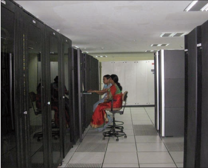
Inside the Data Centre
