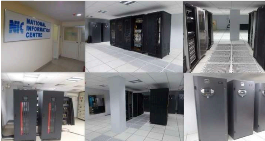
▼ Fig 2.5 NIC West Bengal State Data Centre
